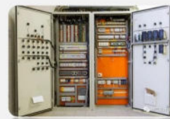
Electrical Cabinet Environmental Monitoring
