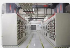
Environmental Monitoring of Power Distribution Rooms
